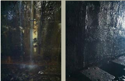
Common drainage problems in tunnels.
