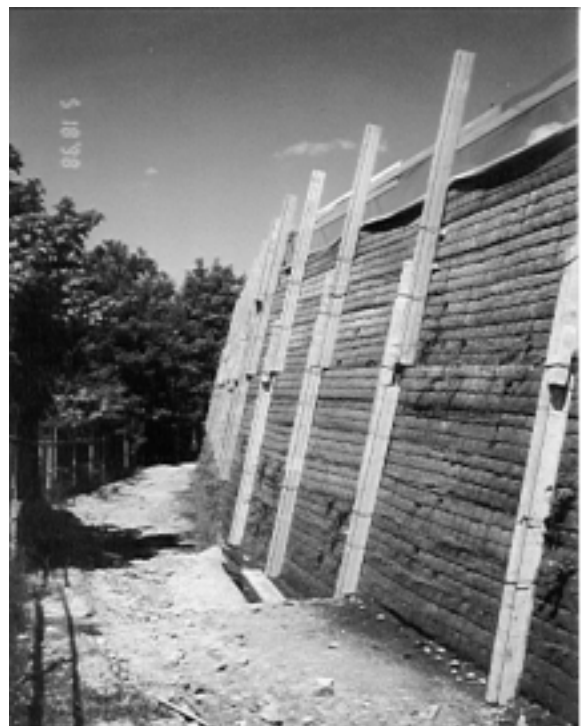
Figure 4: Safety railing and inclination guides
