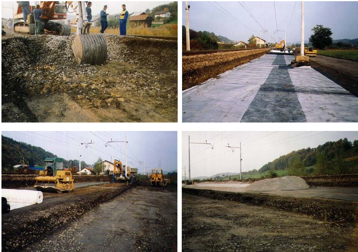
Fig. 5 Excavation, of the existing embankment, installation of the geotextile and geogrid layers, filling and compaction of the new embankment
